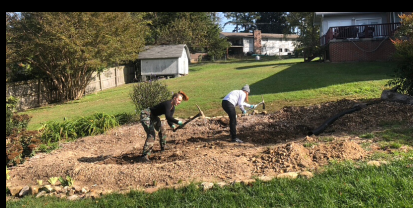
(above) Staff and volunteers dig a rain garden at a Brainerd home.
